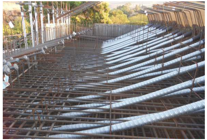
Post-tensioning ducts and anchor heads are placed in the end block. Photo: Eric Matsumoto.
