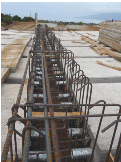
Continuous post-tensioning ducts are spliced at the stiffener beam of the bottom chord. Photo: Eric Matsumoto.
