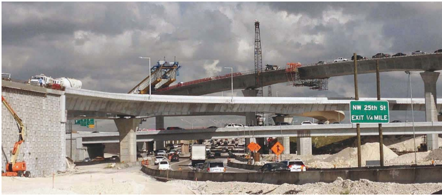
This is a major route to Miami International Airport with more than 430,000 motorists using the interchange daily. Photo: Finley Engineering Group Inc.
