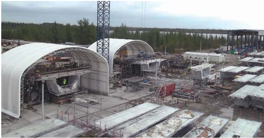
The segment casting yard was located approximately 16 miles away and had two casting cells, which enabled the fabrication of an average of eight segments a week for a total of 783 segments. Photo: Rizzani De Eccher.
