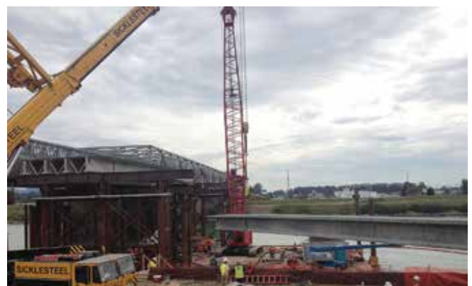
Erection of girders with a 500-ton crane on the river dike and a 200-ton crane on the barge. Photo: Washington State Department of Transportation.
