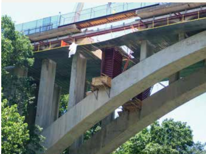
Reconstructing a new column during rehabilitation of the Jacks Run Bridge. Photo: MS Consultants Inc.
