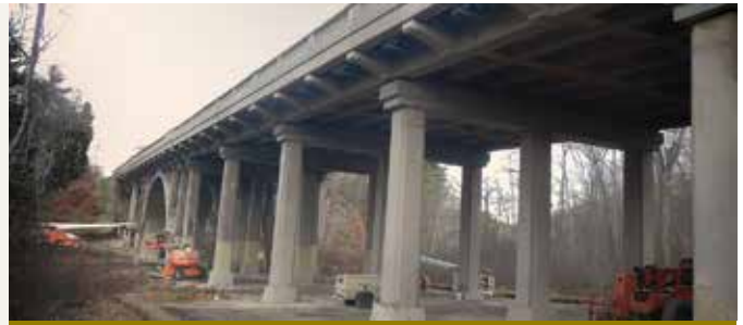
Underside view of the rehabilitated Stillwater Viaduct Bridge. Photo: Vanasse Hangen Brustlin Inc.
