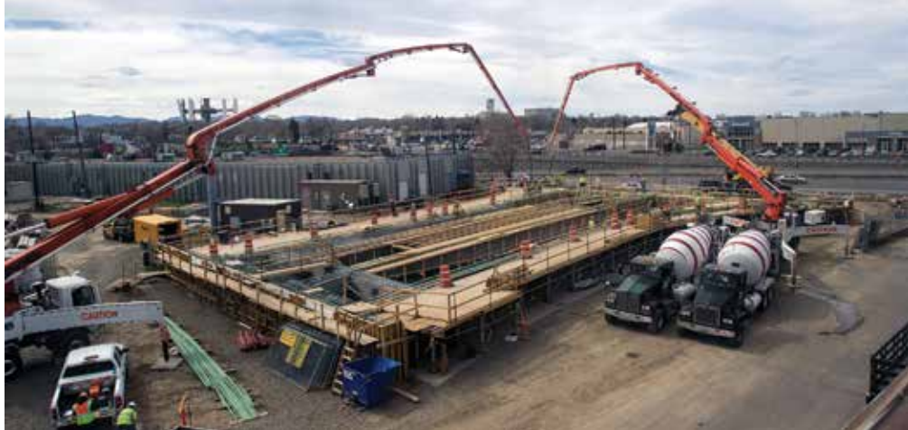
Overview of the bridge staging area (BSA) for the new Pecos Street over I-70 bridge. Photo: 360Media.
