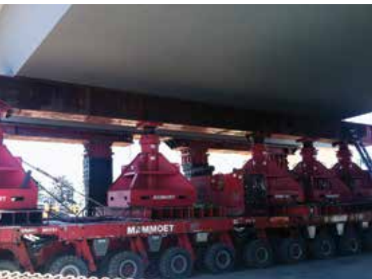
Self-propelled modular transporter equipment installed and ready to move the bridge. Photo: Wilson & Company.
