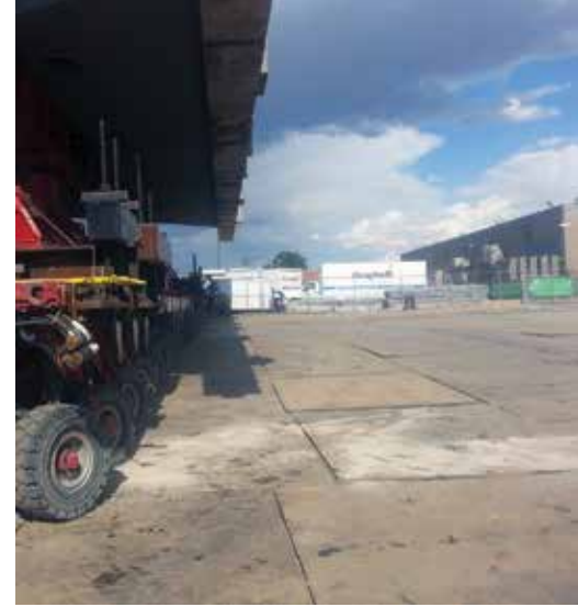
Steel street plates were used to protect travel path surfaces and prevent tires from digging into fill material. Photo: Wilson & Company.
