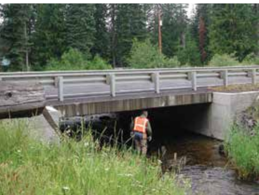
A worker inspects under the State Highway 3 Bridge over Childs Creek in northern Idaho. All Photos: Idaho Department of Transportation
