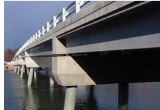
The New Bridge over York River was the first use of the Northeast Extreme Tee (NEXT) beam.
