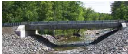
The Brackett Brook Bridge and North Branch Bridge (shown here) in the Carrabassett Valley had to be rebuilt quickly following their destruction in 2011 by Hurricane Irene. Completed on a CM/GC basis, different concrete designs were used for each based on materials available for fastest construction. They were reopened in less than three months. Photo: Maine Department of Transportation.
