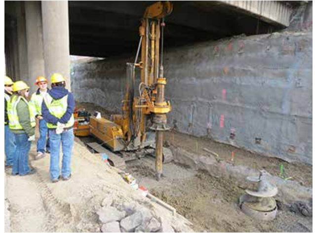
Low overhead caisson drill rig used to construct abutment foundations. Photo: Wilson & Company.
