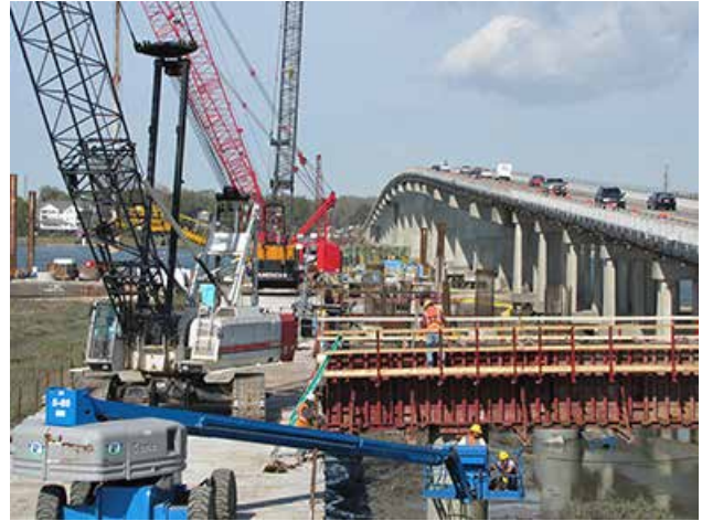
Bridge foundation work being performed from contractor's top-down work trestle. Photo: United Contractors.
