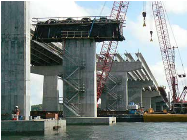
New hammerhead piers and caps being placed in advance of beam setting operations. Photo: Collins Engineers Inc.
