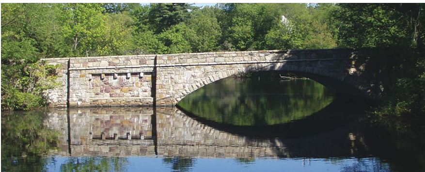
The original, single-span, reinforced concrete spandrel arch Willow Street Bridge. Photo: Matt Hopkinson.
