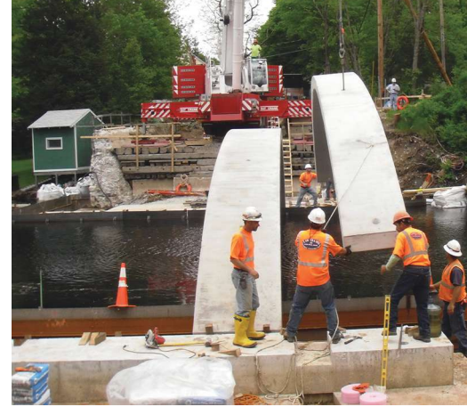
Installation of the precast concrete arches for the Willow Street Bridge. Photo: Matt Hopkinson.
