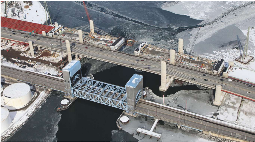
Figure 1. Aerial photo of the southbound main span unit of the Pearl Harbor Memorial Bridge during winter construction conditions. Photo: Connecticut Department of Transportation.
