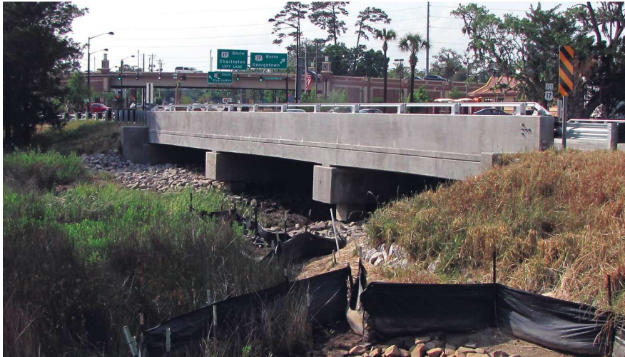
Side view of Bowman Road Bridge over Shem Creek (U.S. Route 17 Overpass in background). All Photos: Adam Lansing.
