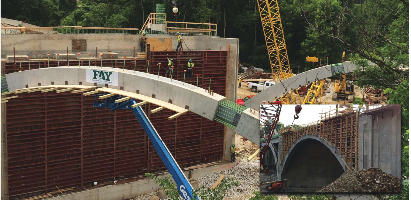
The concrete arch façades for the Frederick Avenue Bridge were manufactured to closely resemble the design of the existing two-span, closed-spandrel filled arch structure that was built around 1930. Photo: Joseph B. Fay Company.
