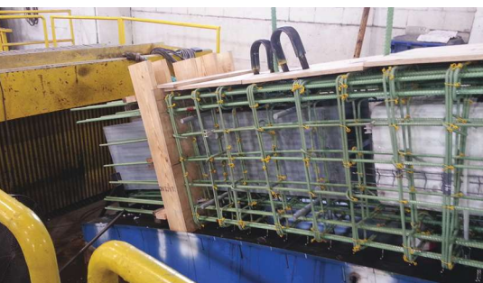
Close up of structural steel splice plate connection ready to be cast into one of the precast concrete box beams.
