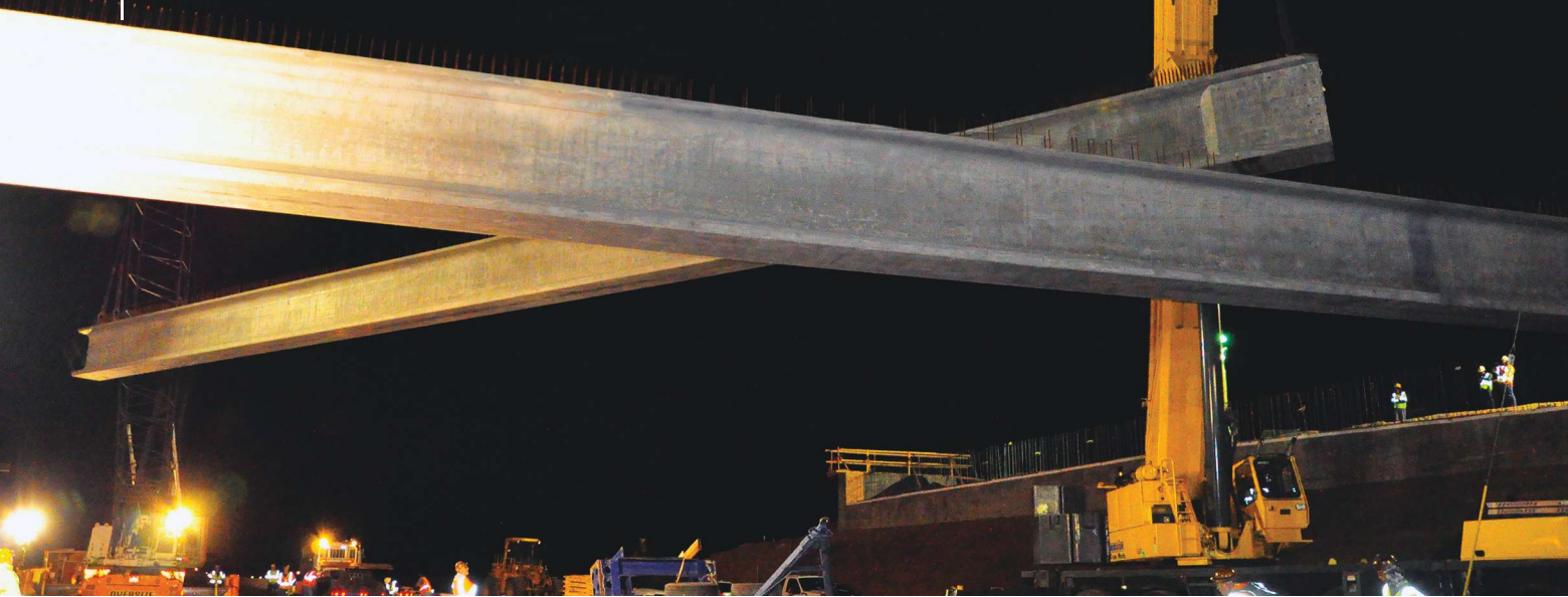
Positioning of the second wide-flange precast concrete girder for placement at the Riego Road Overcrossing. Photo: Brandi Matteoni.
