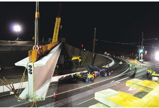
Setting the first of 14 California wide-flanged girders into the second span. Extensive shear reinforcement is required for the girder-slab connection adjacent to the bent cap so that the integral bent cap behaves as desired during a seismic event. Photo: Brandi Matteoni.
