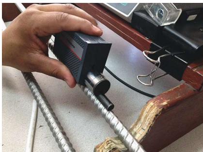
Measurement of steel surface roughness to ensure adequate surface area for coating bonding. Photo: Western Coating Co.
