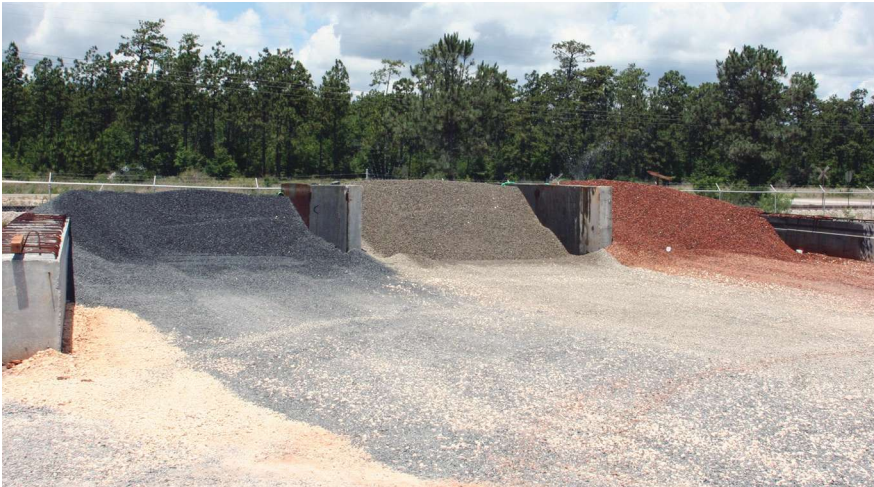
Lightweight aggregate stockpiles at precast concrete plant. All Photos and Figures: FHWA.
