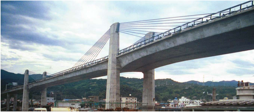
The Odawara Port Bridge, Japan, is the world's first extradosed prestressed concrete bridge, completed in 1994. Photo: Steven Stroh.
