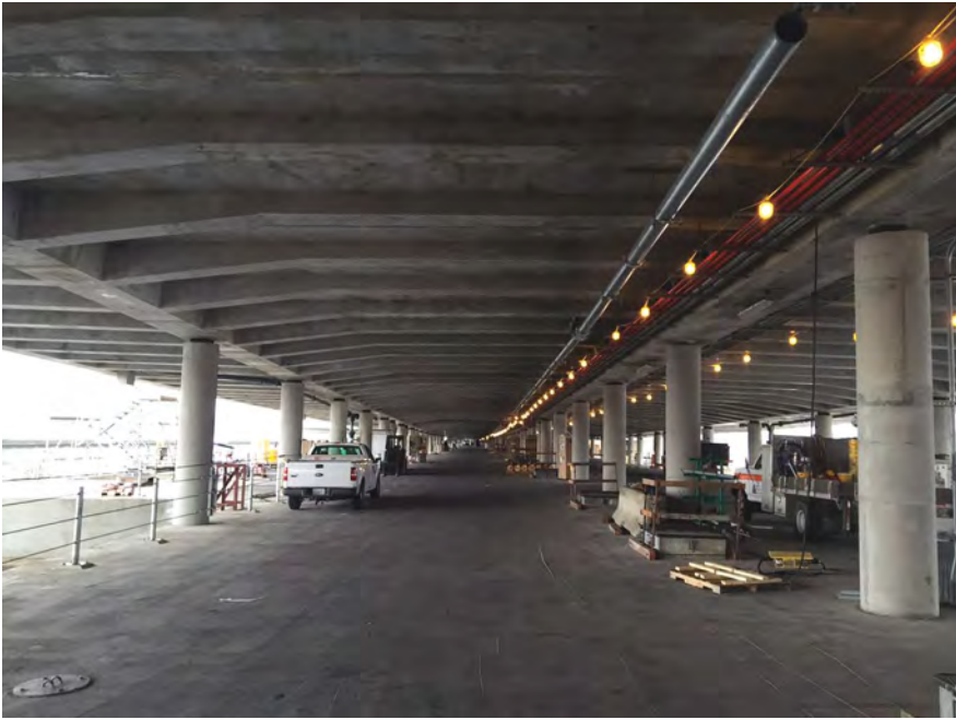
View of completed precast concrete ribbed-slab structure from the top of the pontoon. Photo: International Bridge Technologies Inc.
