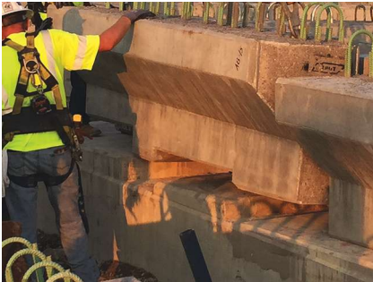
Placing precast concrete end wall on existing pier to make the new abutment. All Photos: Gresham, Smith & Partners.
