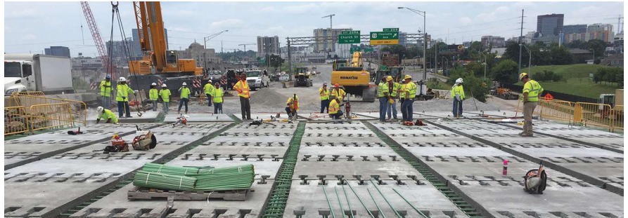
Precast concrete deck panels with longitudinal joints over box beams and splice bar connections between panels.
