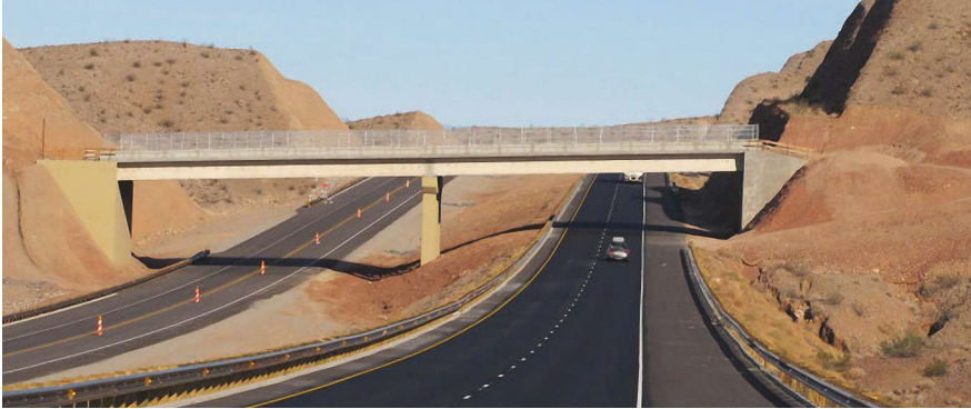
Elevation view of the US 93 Wildlife Overpass Bridge. Photo: Arizona Department of Transportation.
