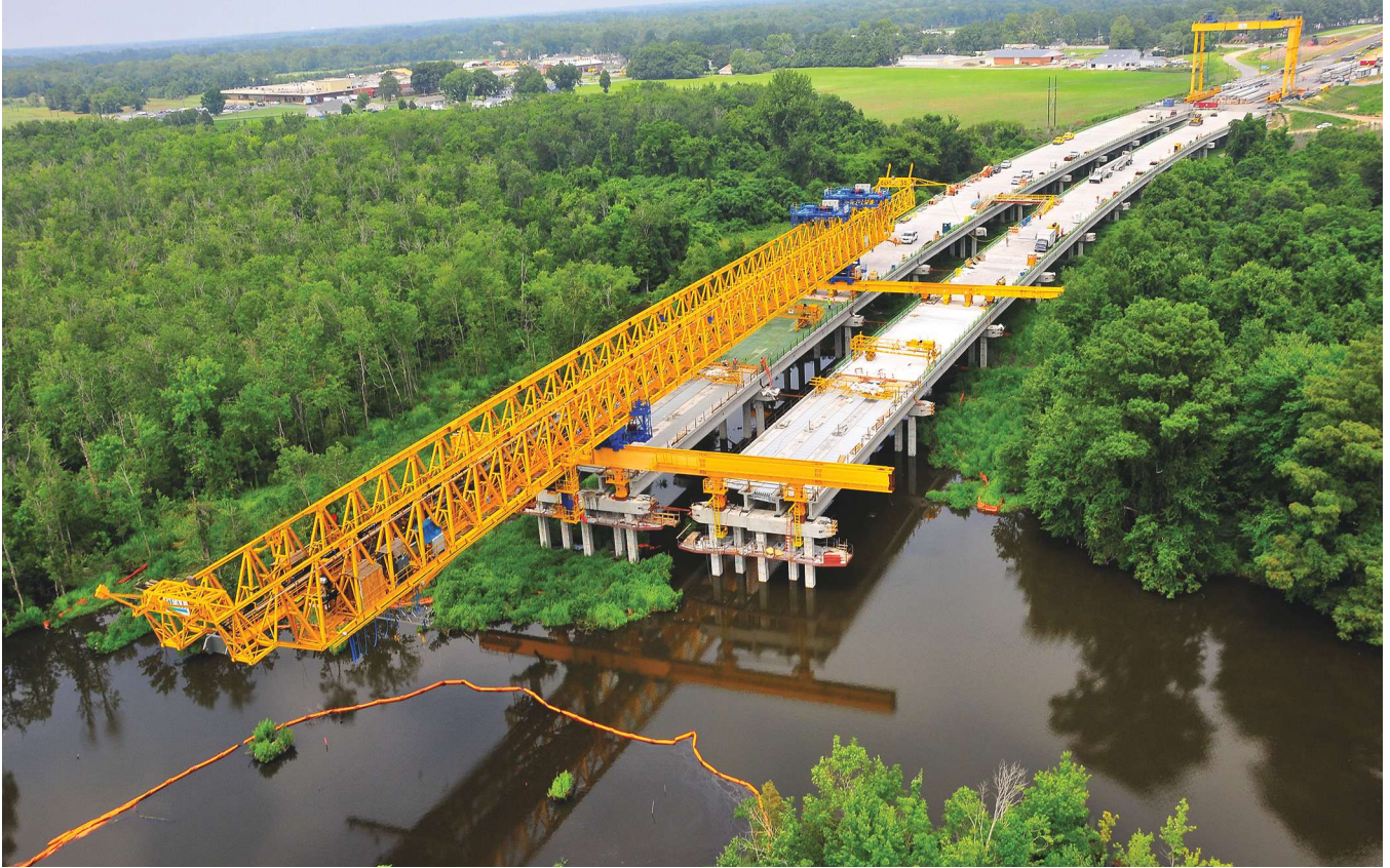
One of the first projects completed using the design-build delivery method in the state was the US Route 17 Washington Bypass bridge in Beaufort County, N.C. It was completed using a gantry system that drove piles, set precast concrete bents, and erected beams from above to minimize impact to the wetlands below. Photo: Flatiron.
