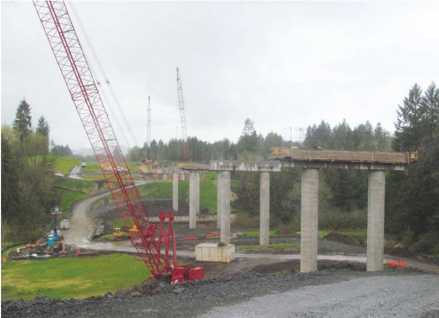
Chehalem Creek Bridge used for comparison of Grade 60 and Grade 80 reinforcement for 8-ft-diameter drilled shafts. All Photos and Tables: Oregon Department of Transportation.
