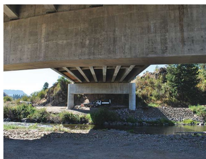
The Indian Creek Bridge used for comparison of Grade 60 and Grade 80 reinforcement for the reinforced concrete crossbeams.
