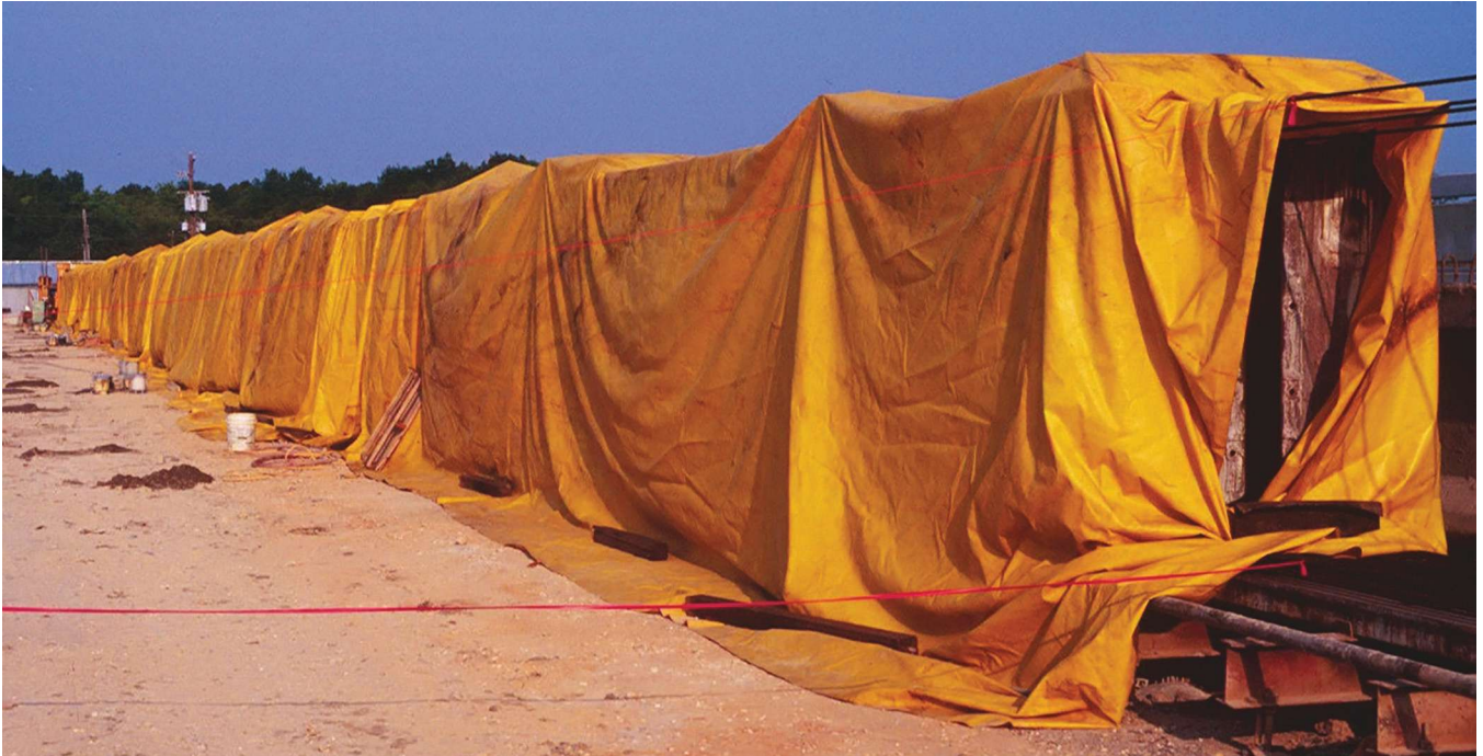
Steam curing of precast, prestressed concrete beams. Photo: Henry G. Russell Inc.
