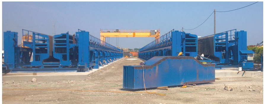
Two side-by-side beds with Nebraska (NU) beam forms. Note the stressing head in the foreground. Photo: e.Construct.USA LLC.
