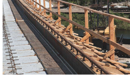
Forms for deck paving and rail for paving equipment create eccentric loading on exterior girder. Photo: Atkins.
