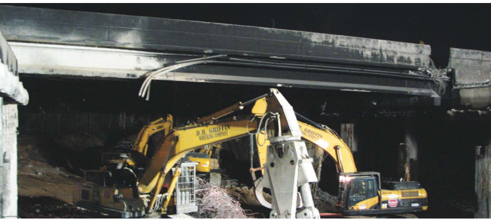
Evaluations found that three spans in each direction needed to be replaced as well as four bents, with round columns and inverted-tee bent caps. Demolition of the spans began immediately. All Photos: Georgia Department of Transportation.
