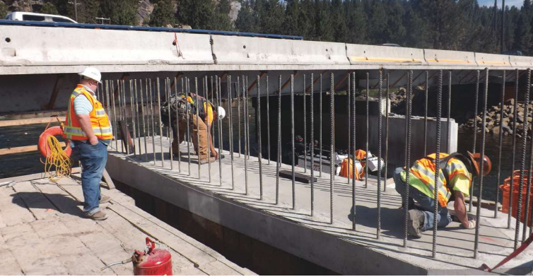
Stage 1 upper pier segment erected. Workers are placing temporary bearings for deck girders. Projecting vertical bars will be cut at deck girder locations.
