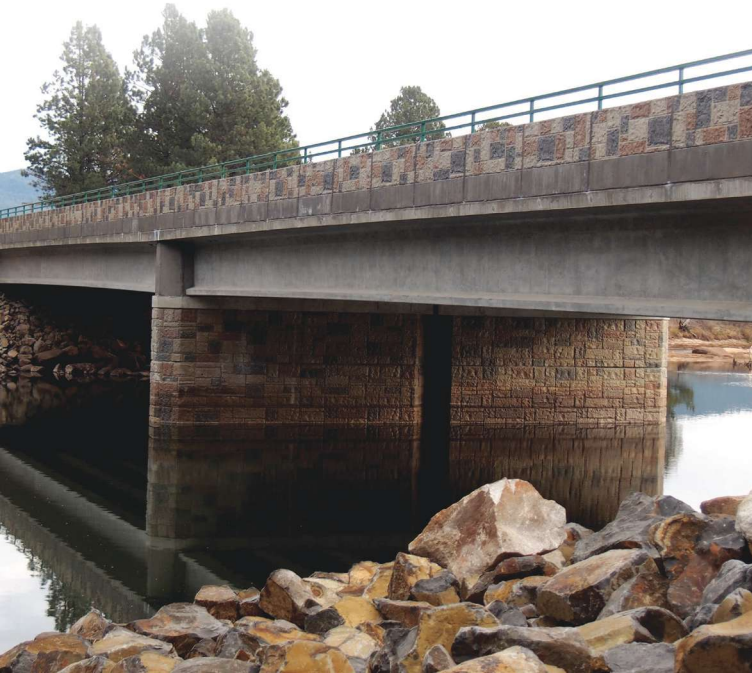
Completed bridge with concrete barriers and piers stained to match local stone. All Photos and Figures: Idaho Transportation Department.
