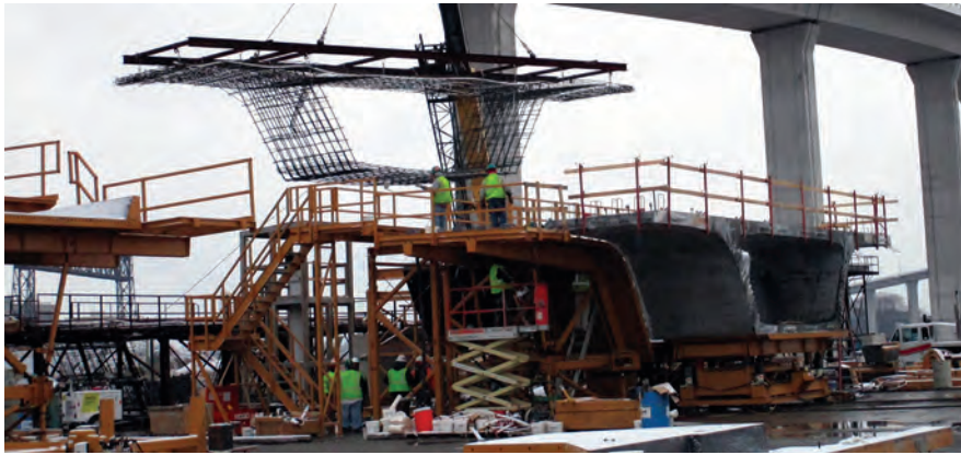
Figure 4. ASTM A1035-CS alloy reinforcement cage being placed in a segment form for the Lesner Bridge in Virginia Beach, Va.
