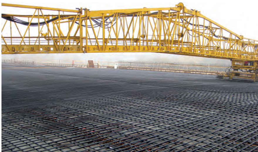
Figure 5. Deck for Circle Drive Bridge in Saskatoon, Canada, with conventional Grade 60 reinforcement replaced with ASTM A1035 CS Series 9100.
