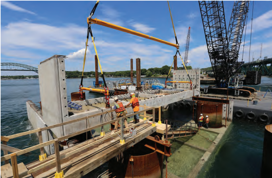
Precast concrete tubs for forming the footings on the Sarah Mildred Long Bridge provide both short-term and long-term benefits.
