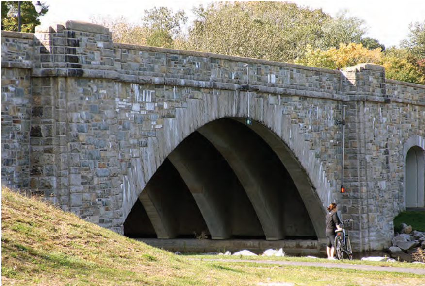
The Humpback Bridge over the Boundary Channel on the George Washington Parkway near Washington, D.C., consists of a single span with segmental precast concrete arches.
