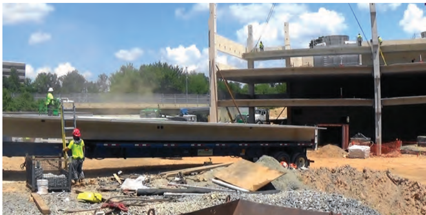
A rigger prepares for installation of a precast concrete element in a common jobsite area. All Photos: Law Office of Adele L. Abrams PC.
