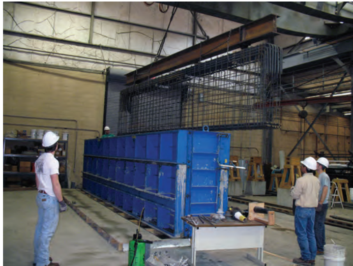
Students in the Ferguson Structural Engineering Laboratory at the University of Texas at Austin observe a reinforcing bar cage being placed into a form. Photo: David Birrcher and Robin Tuchscherer.
