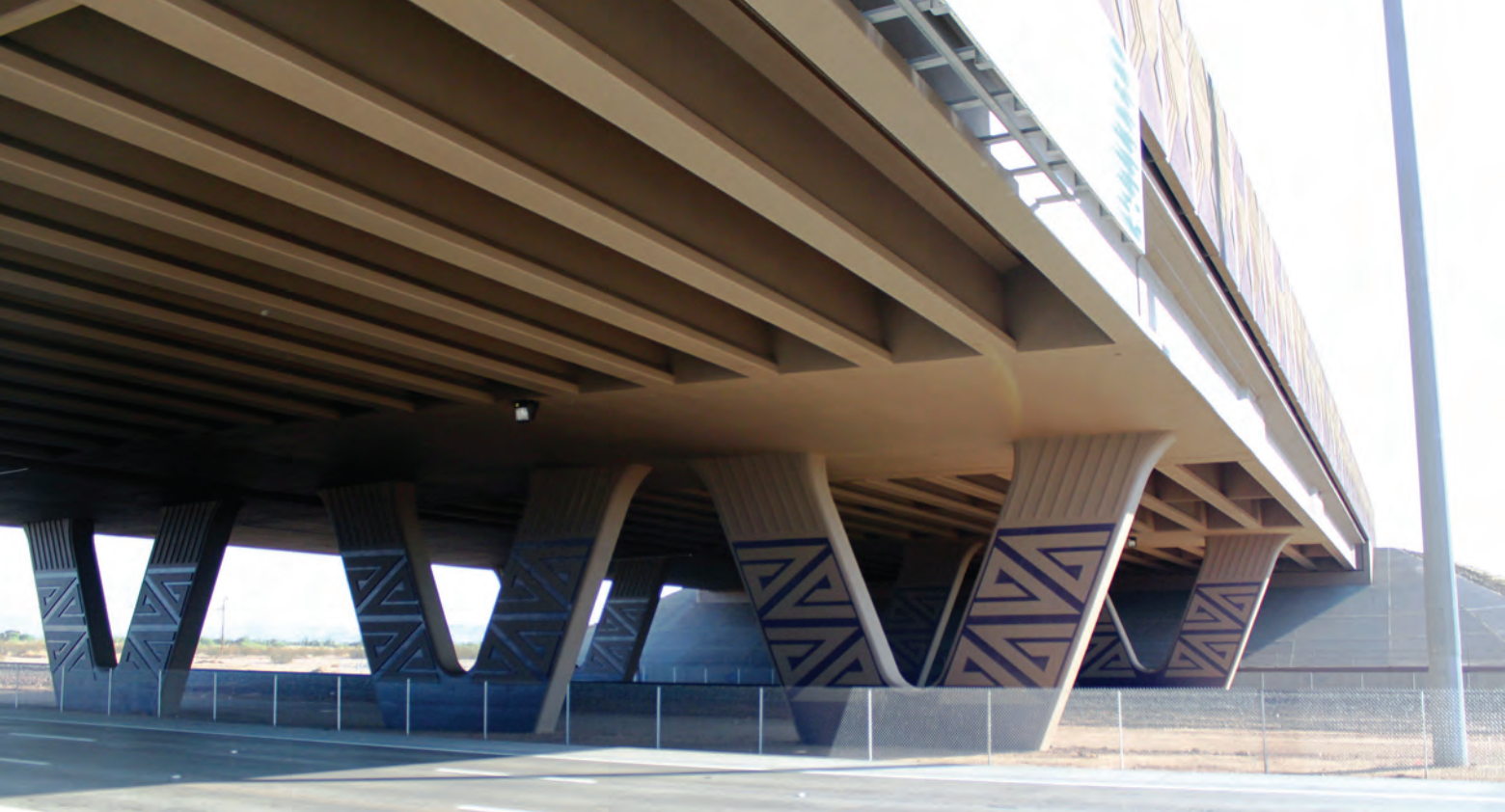
Completed piers 2 and 3 showing Y-shaped columns and the interface of the cast-in-place concrete pier tables with the precast concrete girders. Photo: Stanley Consultants.
