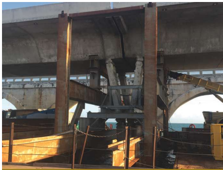
Temporary support system in place and removal frame installed on existing V-pier. Jacking system can be seen.
