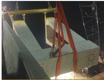
V-pier being lowered from Long Key Bridge to the construction barge at night. Note holes for dowels to drilled shafts.
