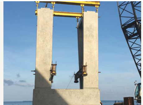
New V-pier being lifted and placed onto the temporary support system. Hydraulic jack and roller assembly is mounted on the column legs.
