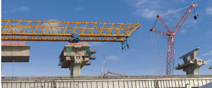
Gantry erection of cantilever at expansion pier and split-pier segment erection by crane.
