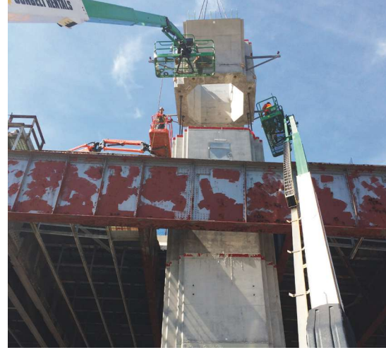
Erection of precast concrete column segment. Column location constrained by existing edge girder.
