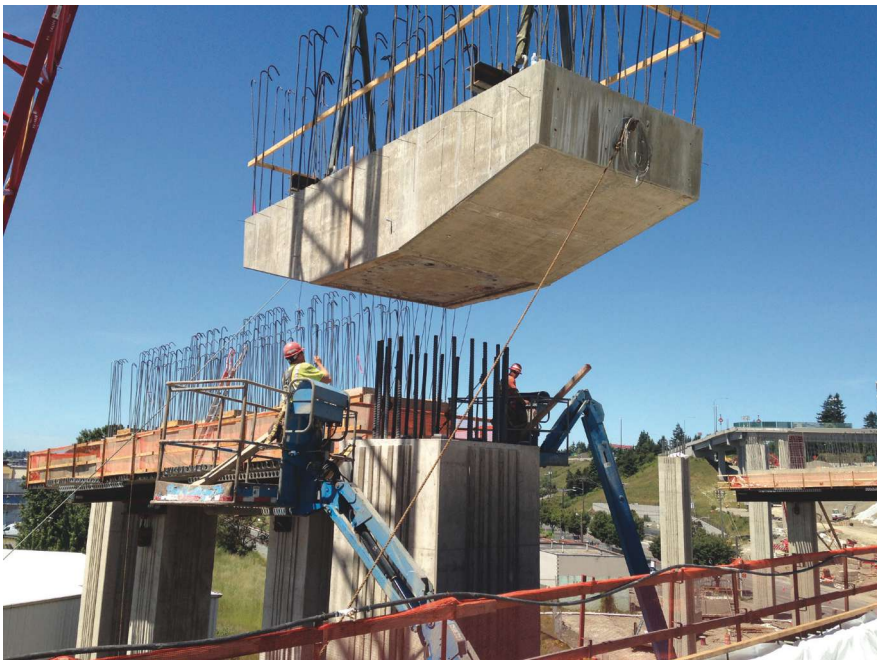
Erection of precast concrete crossbeam at Nalley Valley Interchange, Tacoma, Wash.. Photo: Geoff Swett, Washington State Department of Transportation.
