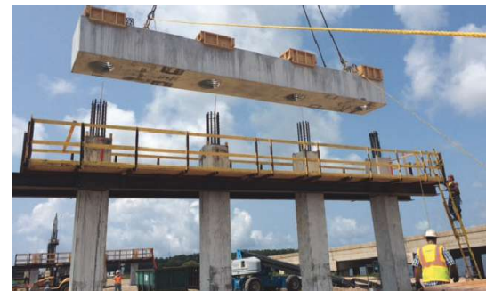
Precast concrete bent cap being erected on SR 83 (US 331) over Choctawhatchee Bay. Photo: WSP.
