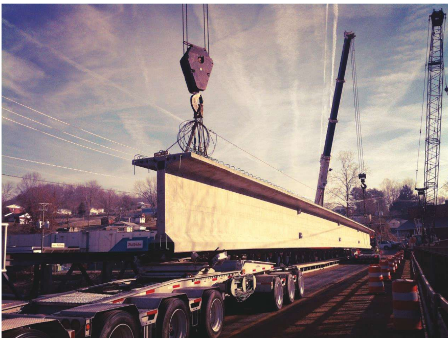
The concrete beams of the Coopers Creek Bridge were long and would have been heavy, but the design-build team specified lightweight concrete to both reduce the weight and minimize the crane size.
