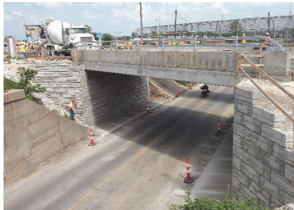
Simple span prestressed box sitting on geo-synthetic reinforced soil abutments in Missouri.
