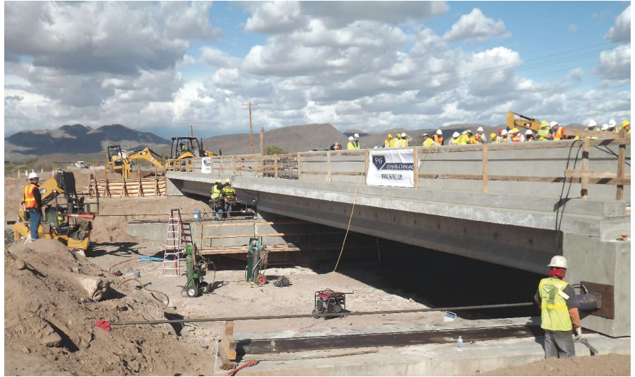
Two span bridge slid into place in Arizona using steel on steel with grease for the slide system. All Photos: Finn Hubbard.
