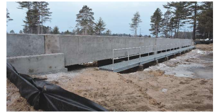
Three span prestressed box bridge built during the winter of 2015 in Upper Michigan.
