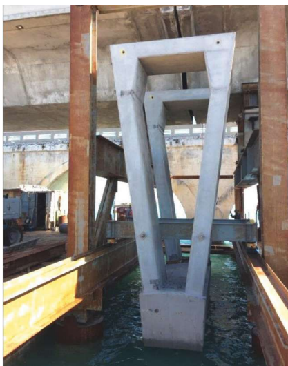
New pier seated in temporary support system and ready for side launch into permanent position. Photo: FDOT.
