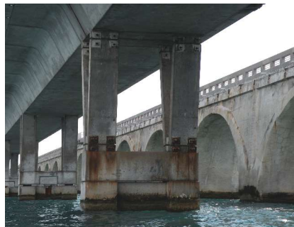
Photo of the existing V-pier with the 1908 arch structure in the background. The galvanized compression plates installed shortly after construction are visible. Photo: Luis Vargas.
