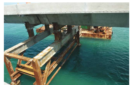
Temporary support system spanning between temporary outboard drilled shafts supporting the bridge after the V-pier has been removed. Photo: FDOT.
