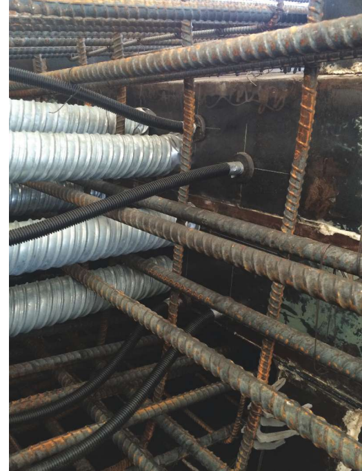
Reinforcing bar cage, grouting tubes, and steel duct for connection between drilled shaft and replacement pier. Photo: Kurt Podoll, Standard Concrete.
