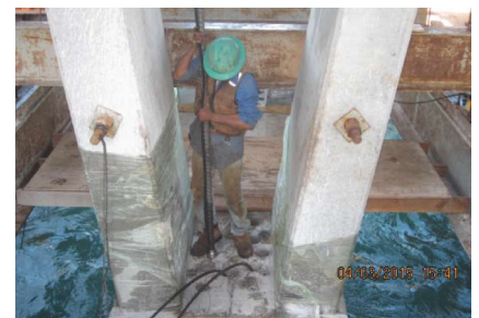
High-strength bar installation and cementitious grouting operations using ABC connection details. Photo: FDOT.
