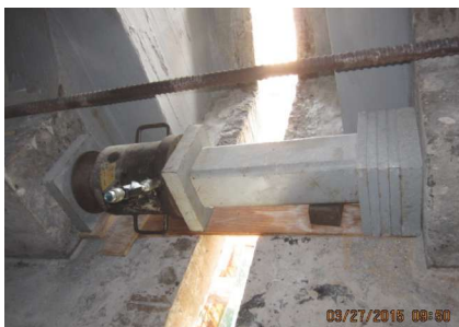
Temporary devices used to lock expansion joints during pier replacement. Photo: FDOT.
