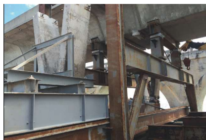
Temporary support system supporting spans as existing V-pier is being removed. Photo: FDOT.
