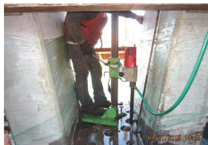
With the new V-pier in position, anchor holes were used as drilling template for establishing connections into drilled shaft. Photo: FDOT.
