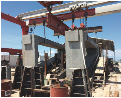
Special lifting and handling procedures were established. Photo: Kurt Podoll, Standard Concrete.
