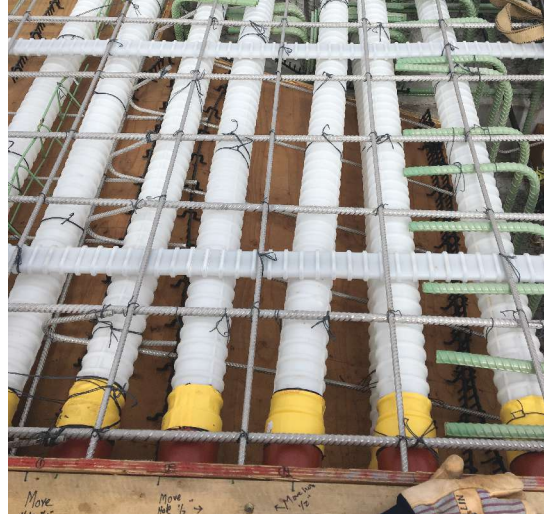
A cast-in-place pier table segment on an approach bridge. The round longitudinal post-tensioning ducts are 4 in. in diameter, and the flat transverse post-tensioning ducts are 1 in. by 3 in. Photo: Parsons Transportation Group.
