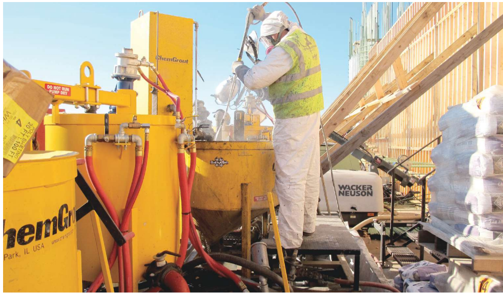
Grout being batched in a colloidal mixer. Photo: Paul Kivisto, Minnesota Department of Transportation.
