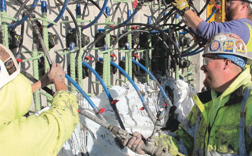
Grout being pumped into the ducts at the crossbeam in the extradosed spans (the crossbeam connects two columns of a pier). The crew is grouting the post-tensioned bars that extend across the width of the crossbeam (about a 16-ft-long bar). Photo: Paul Kivisto, Minnesota Department of Transportation.
