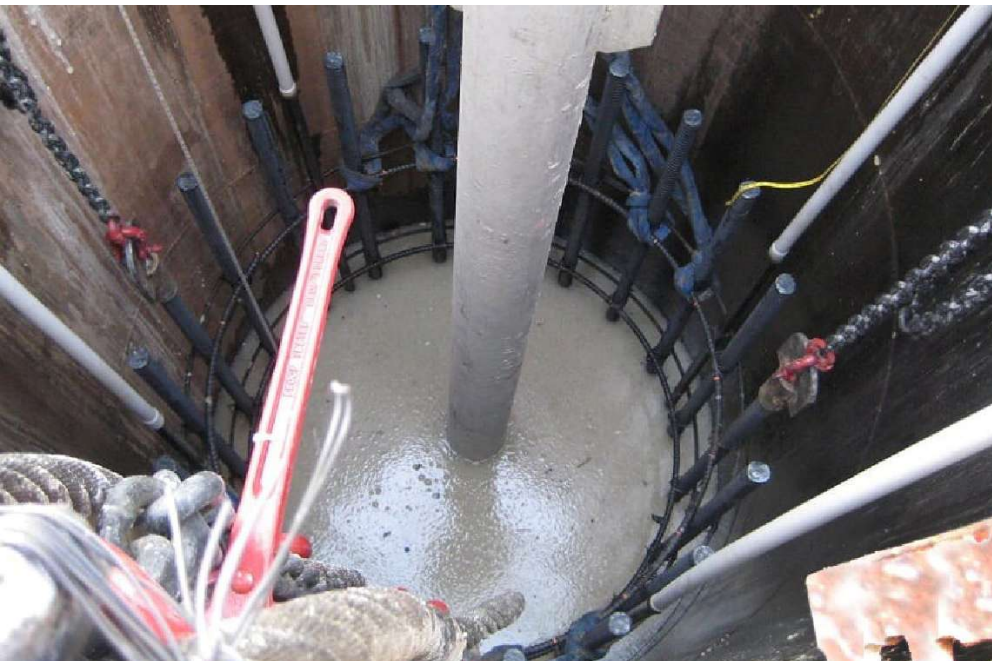
Tremie being used for concrete placement for a drilled shaft. All Photos: Federal Highway Administration.
