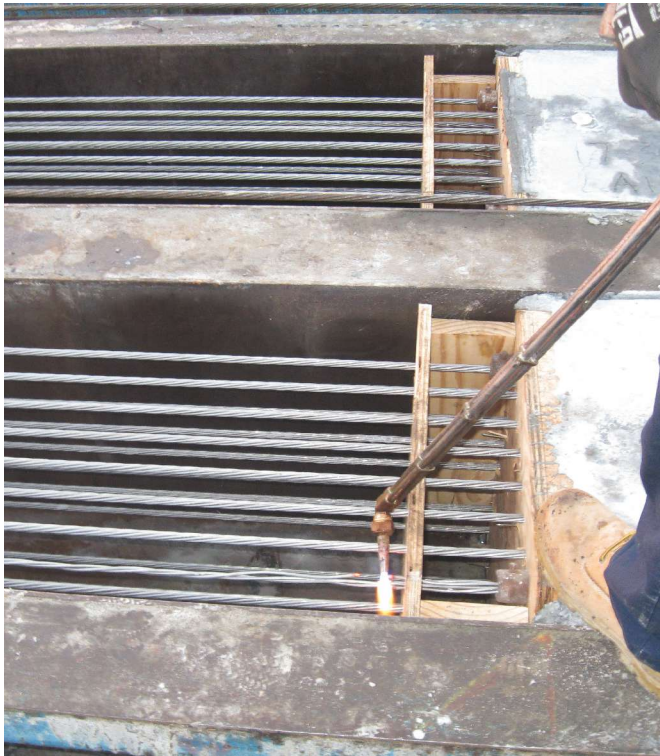
The normal de-tensioning procedure was used, but workers reported that more oxygen was needed in the gas mixture to flame-cut the stainless steel strand than carbon steel strand.
