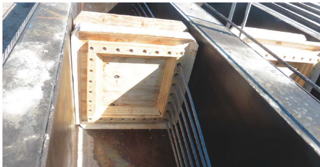
A custom header to separate the piles in the casting bed was fashioned to form the 2-in.-deep recess for strand. This formwork was challenging to make and remove.
