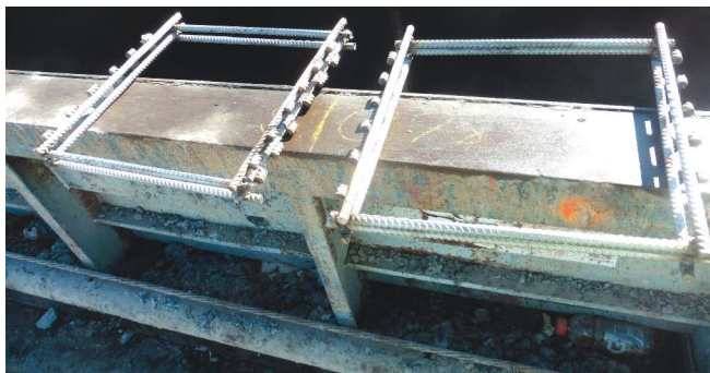
Gulf Coast Pre-Stress typically uses a template made from reinforcing bars to keep strands in position in the middle of long piles. For this project, the template had to be stainless steel.
