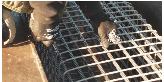
Stainless steel preformed wire ties were used to tie the spirals to the strand. Workers reported that the stainless steel ties required more effort to tie than their carbon steel counterpart.
