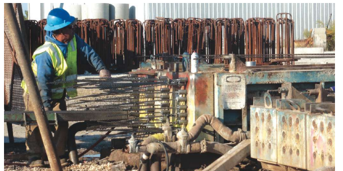
No modifications to the tensioning procedure were necessary for the stainless steel strand.
