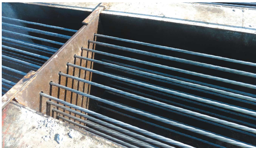
Stainless steel strands being used in the production of prestressed concrete piles for Louisiana Department of Transportation and Development Bayou Thunder Overflow Project (LA 1 bridges near Grand Isle). All Photos: Krista Brown.
