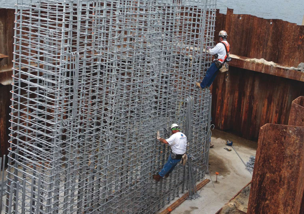
Galvanized reinforcement cages were assembled on barges and lifted into place, extending up and out of the sheetpile cofferdams.
