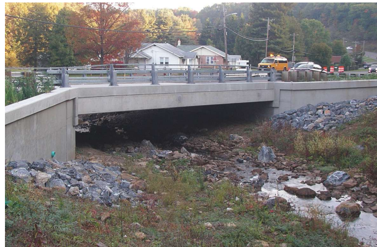
Bridge No. 01011 – Maryland Route 36 over Elk Lick Run. Photo: Maryland Department of Transportation State Highway Administration.
