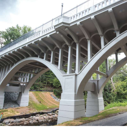
Bridge No. 15033 – Maryland Interstate 195 over Sligo Creek Parkway and Sligo Creek. Photo: Johnson, Mirmiran & Thompson.
