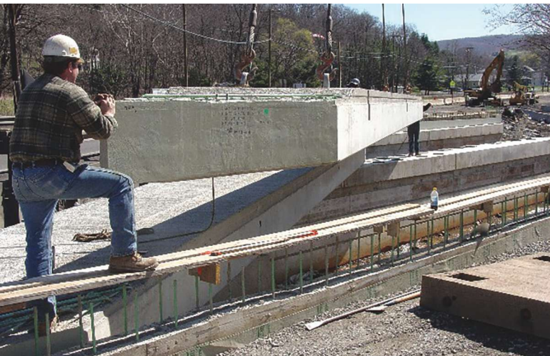
A prestressed concrete solid slab being installed for the Maryland Route 36 bridge over Georges Creek. Solid slabs are the "go to" bridge type in Maryland for spans less than 55 ft. Photo: Maryland Department of Transportation State Highway Administration.
