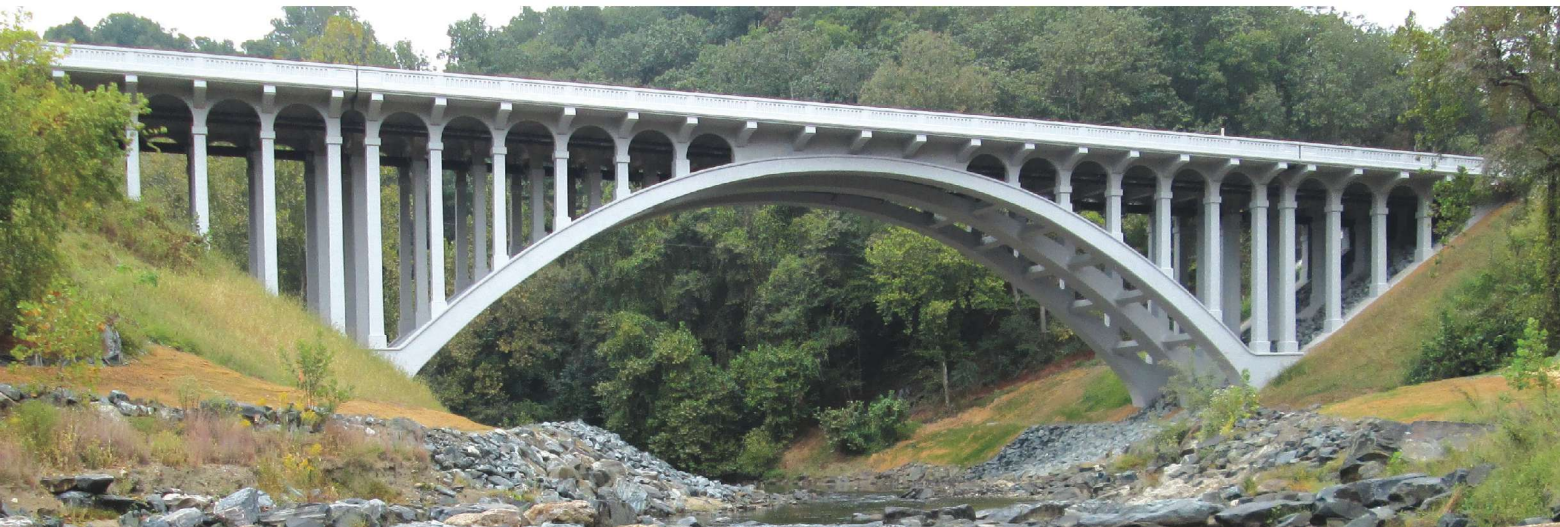
Bridge No. 03109 – U.S. Route 40 over Patapsco River. Photo: Maryland Department of Transportation State Highway Administration.
