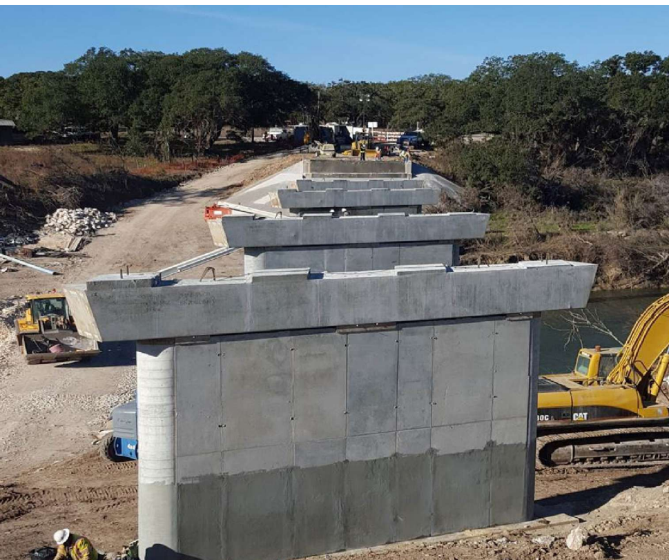
Prestressed, precast concrete bent caps (PPBCs) at Fischer Store Road in Hays County. The contractor installed all of the PPBCs in one day. Photo: Texas Department of Transportation.
