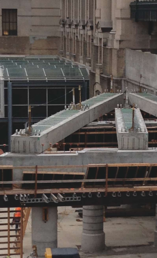
Complex geometry at the Carriage Pavilion end of the bridge required a high level of detail for fabricating box girders and deck form panels.
