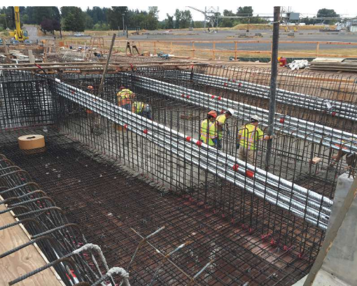
Placing concrete in the bottom slab of a box girder near a pier. Post-tensioning ducts can be seen in the webs. Photo: OBEC Consulting Engineers.
