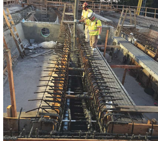
Placing concrete in web of the box girder. Photo: OBEC Consulting Engineers.
