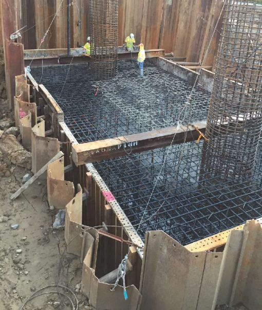
Placing concrete for bent 2 footing. Note the scale of the large footing supporting both columns. Photo: OBEC Consulting Engineers.
