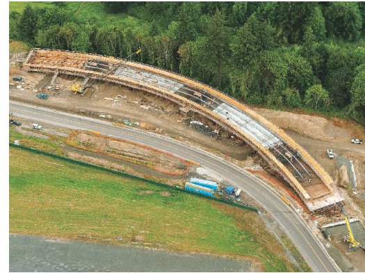
Aerial view of bridge formwork showing horizontal curve of structure. Photo: Oregon Department of Transportation.
