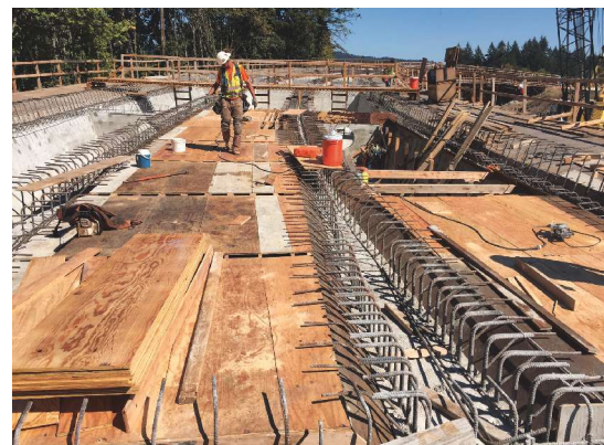
Top slab formwork being constructed. Detailing the reinforcement to avoid interferences and congestion was challenging. Photo: OBEC Consulting Engineers.
