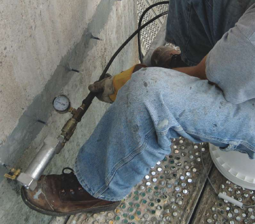
Epoxy injection of cracks using a dual-component pump with positive displacement and metering capabilities. The epoxy resin is delivered through two lines to the static mixer, where it is mixed and immediately discharged into the crack through the injection port.
