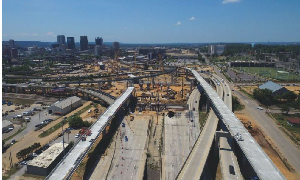
On the Interstate 59/20 Central Business District Bridge replacement project in Birmingham, Ala., Armeni consulted on cost estimates, schedules, and options for construction methods. Photo: Armeni Consulting Services.
