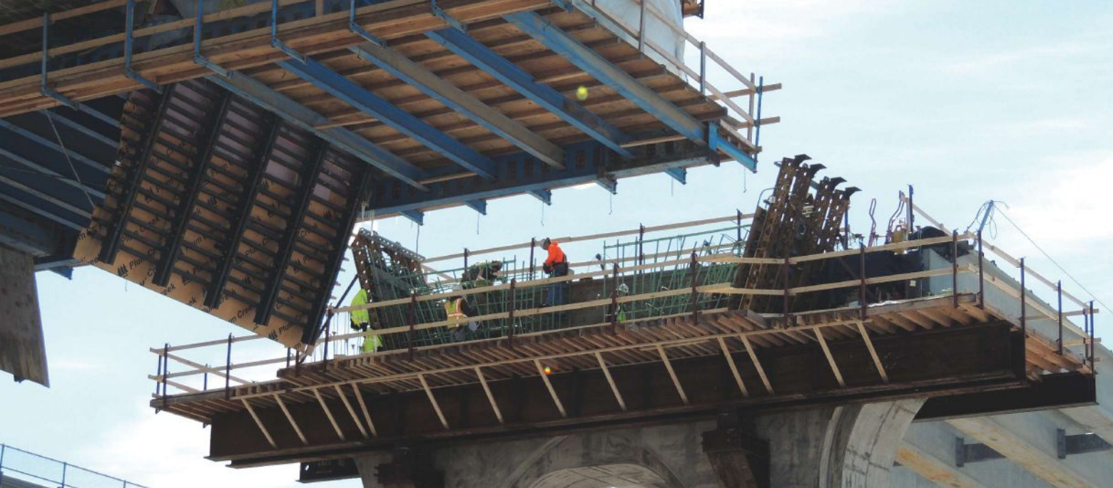
For Bridge 85851 in Winona, Minn., which opened in 2016, Armeni Consulting Services provided independent cost estimates. Photo: Armeni Consulting Services.
