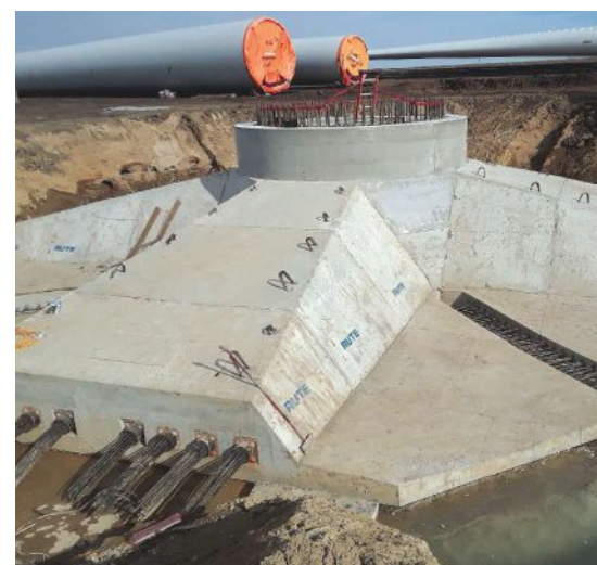
A photo showing the nearly completed base of a wind-turbine tower. Photo: Armeni Consulting Services.
